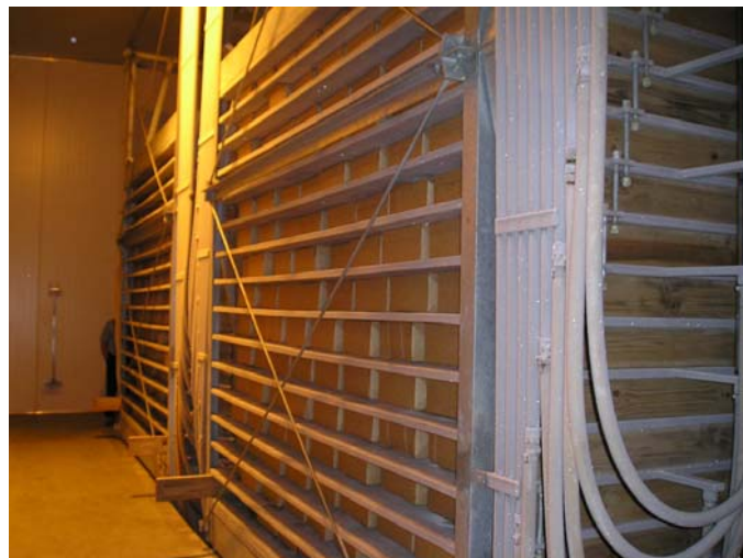
Fig. 10. Plate freezer employing secondary refrigerant – general view
