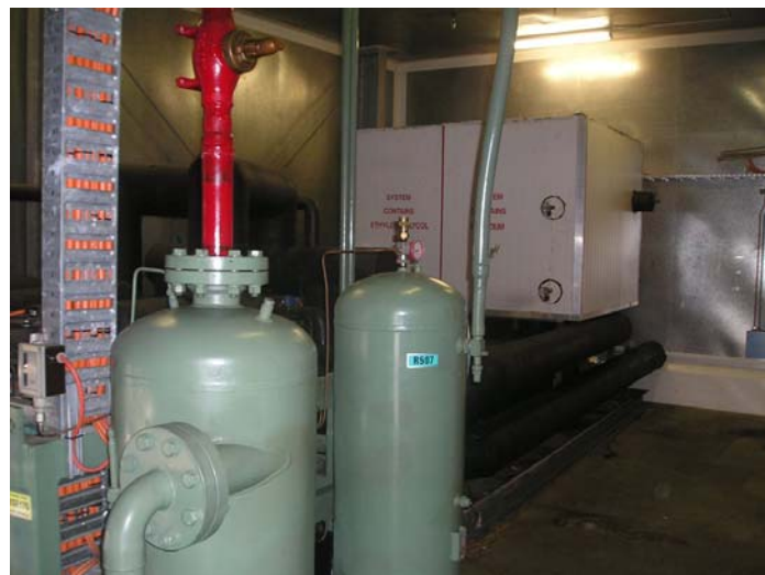
Fig. 12. Plate freezer engine room
